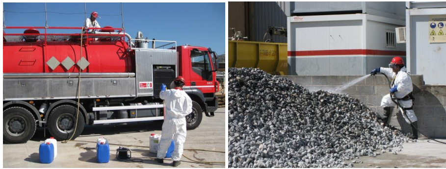
Figure 8. Mixing process of dust suppressant nanopolymer with water and application to the untreated ballast.
